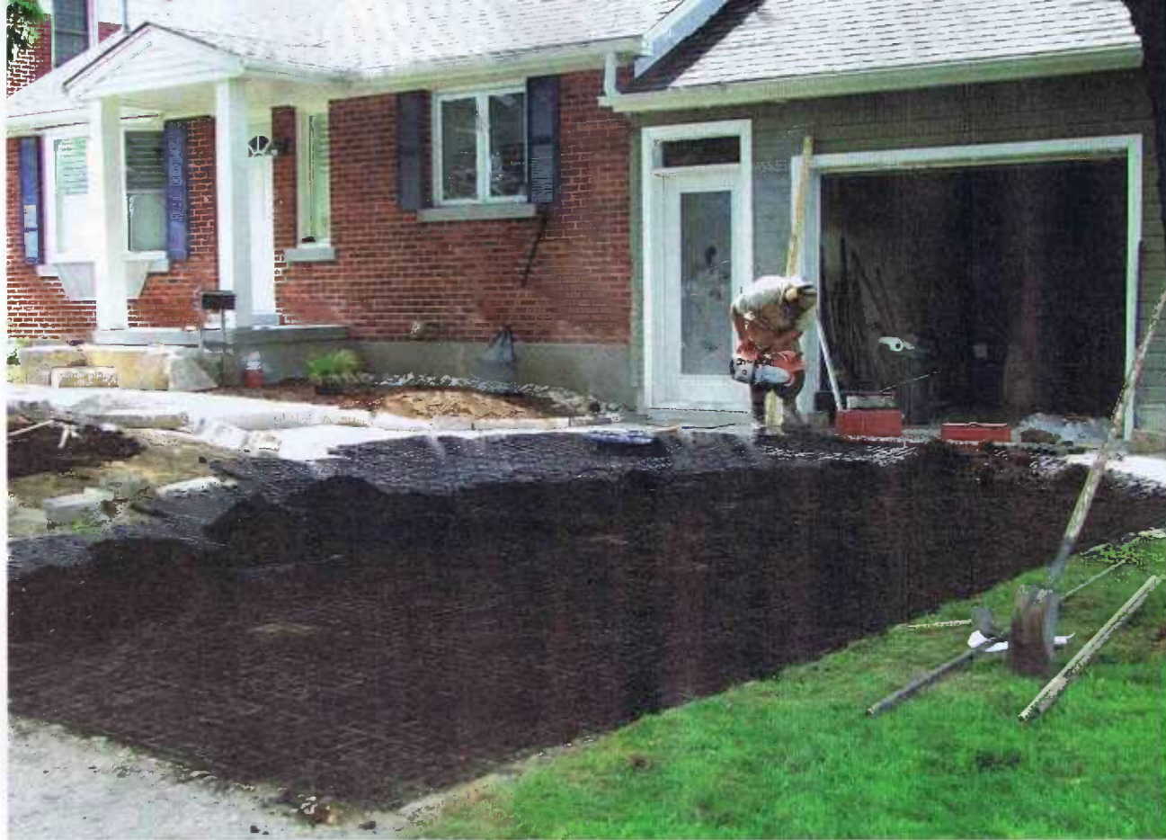
The growing medium is spread. The most important factor in this kind of driveway is getting the foundation level to eliminate run-off.
