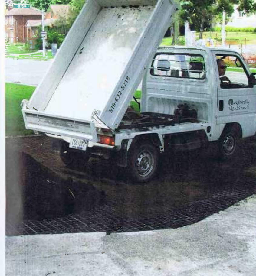
Loads of a compost-and-sand growing medium are poured onto the plastic grids. If a short groundcover is planted, the grid may be visible from the street.
