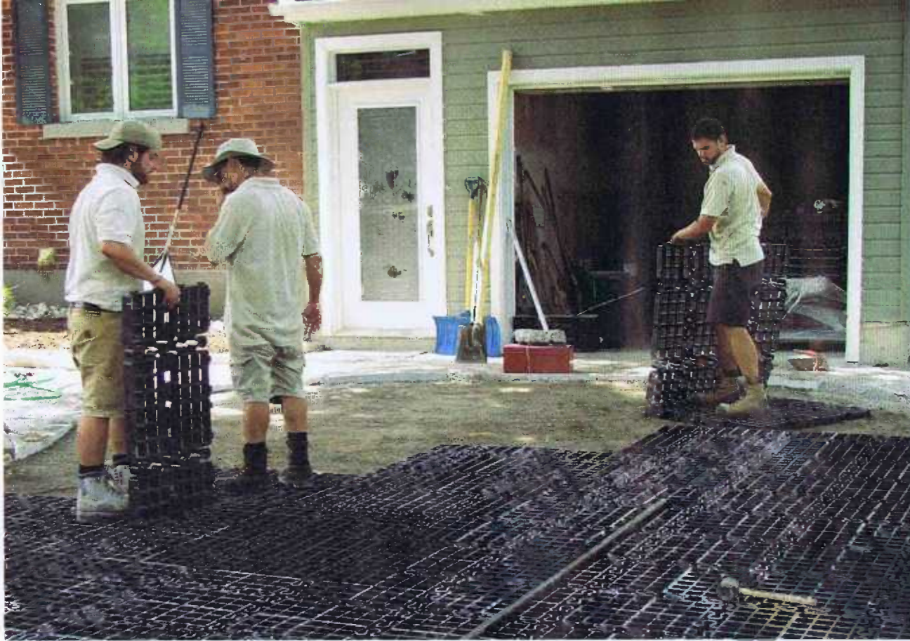
A grid of one-metre plastic squares, made from recycled shrink wrap, are snapped together to form the foundation for the groundcover. The flexible grid isn't as prone to frost-heaving as paving stone driveways.
